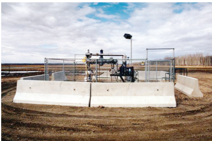
Proper design of the injection scheme is only one part of the picture, however. Operation of the compressor is also crucial. Operators should avoid the temptation to reduce the compressor discharge pressure so that it is merely sufficient for injection. This may lead to problems with the formation of an aqueous phase or a hydrate.
